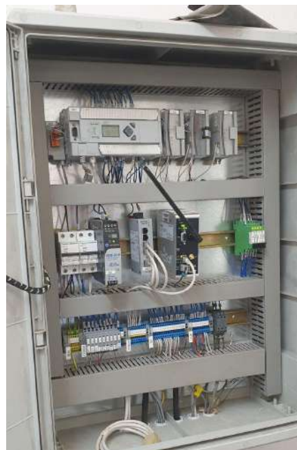
Figure 20: Typical layout of a control cabinet
