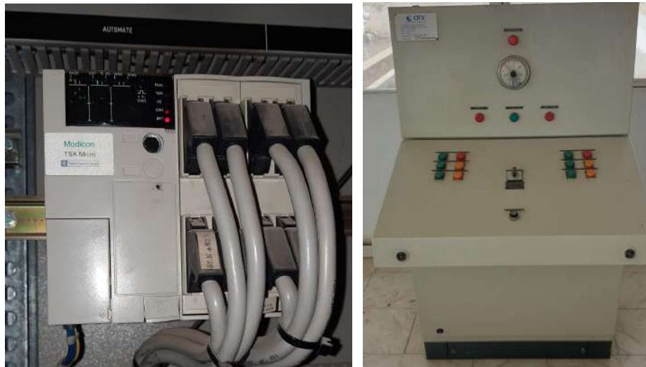
Figure 26: Controller and control desk available on Zahle WTP
