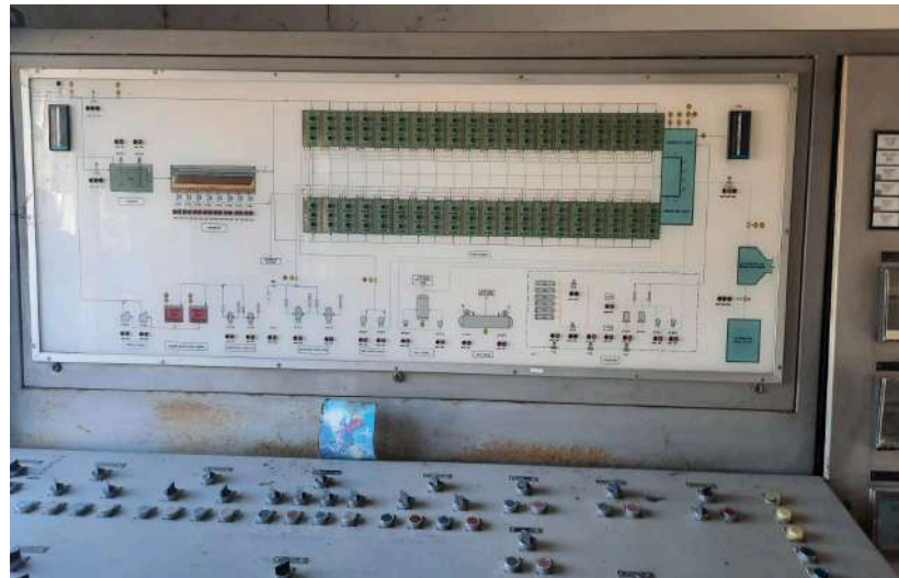
Figure 21 : HMI elements available on Dbayeh WTP
