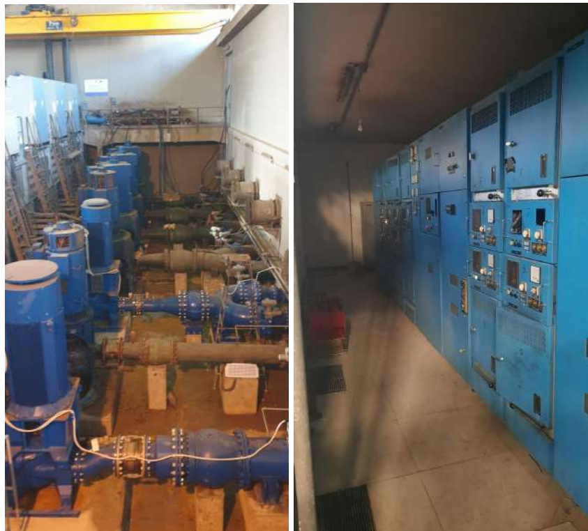
Figure 22 : Pumping lines and switchgear of Dbayeh WTP
