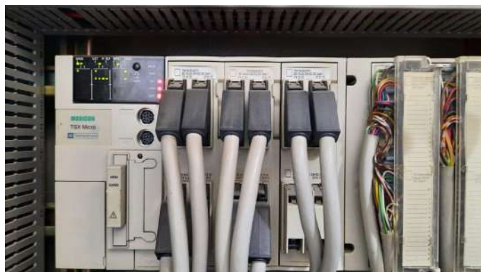
Figure 20 : Jbeil pumping station PLC showing errors
