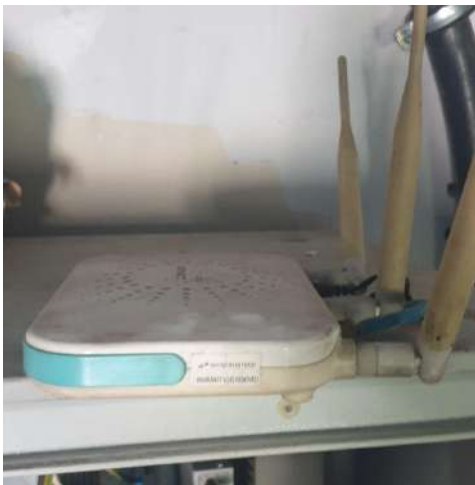
Figure 19 : Added Wifi modem for local supervision
