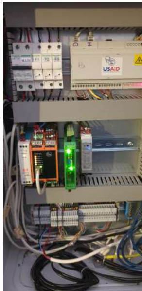
Figure 31: Vibration system panel
