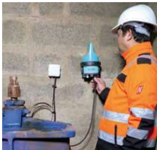
Figure 27: Example of the installation of a self enclosed data logger
